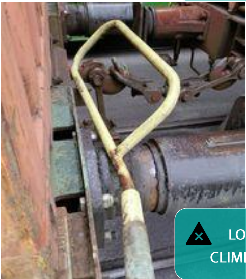
✘ WRONGLY POSITIONED CONTAINER ATTACHMENT
